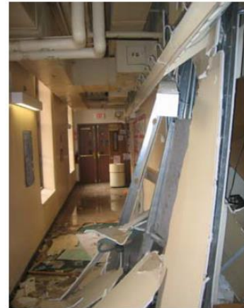
Figure 2 - Hallway Outside Laboratory Showing Explosion Damage
